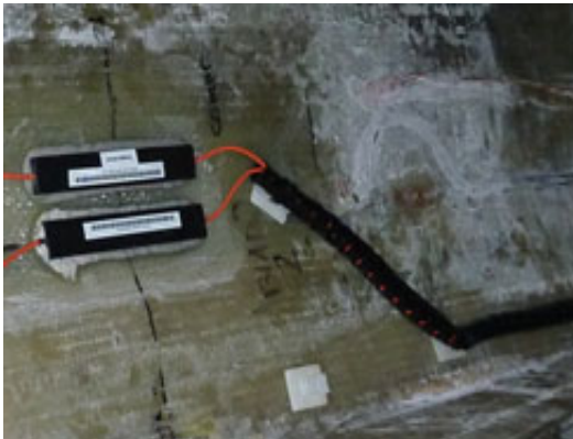
Fig. 2.15 Cable protected with corrugated tubes
