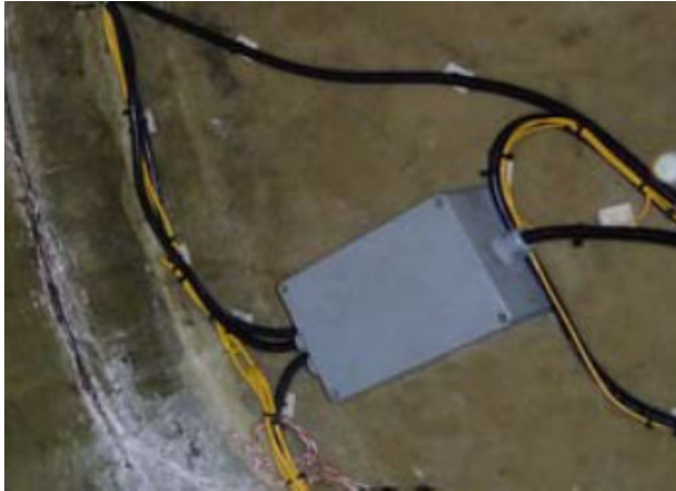
Fig. 2.37 Protection boxes for extra cable and connections
