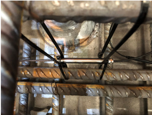
Fig. 2.34 Sensor to be embedded secured in place with plastic cable ties
