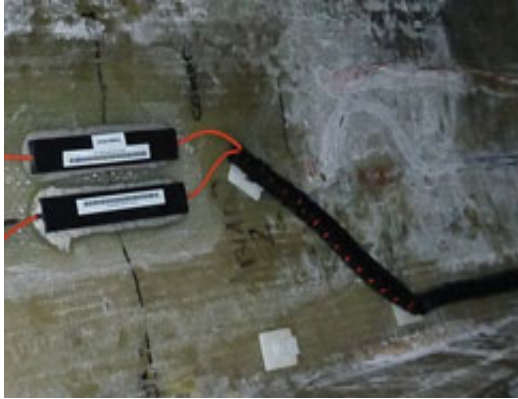
Fig. 2.31 Cable protected with corrugated tubes
