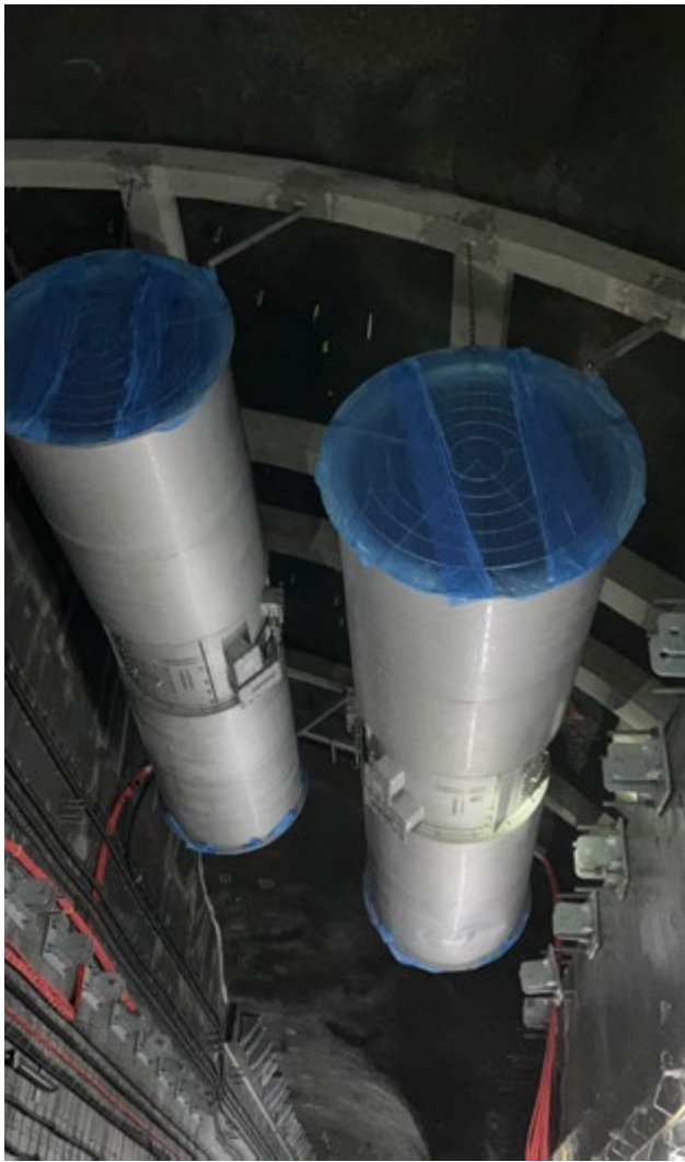
Fans used to aerate train tunnels
